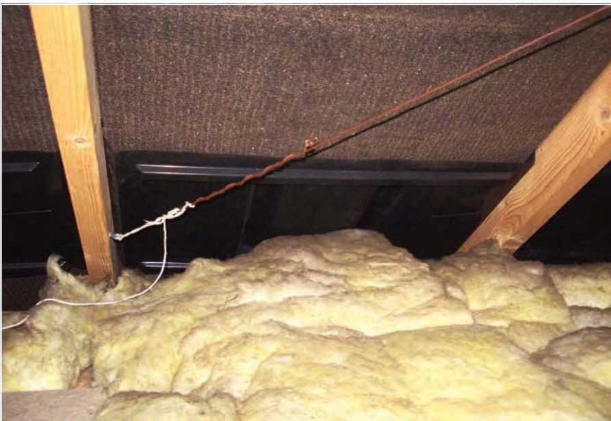
Fig. 8: Looking at the open end held tight with string attached to a roof joist.
