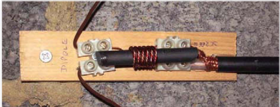
Fig. 5: The balun mounted high in the apex of a gable-end wall.
